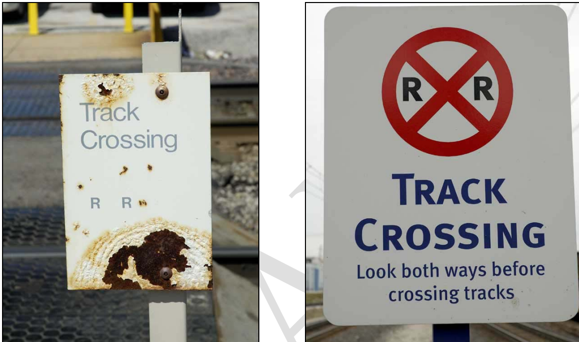
Figure 10: Examples of poor sign maintenance (left) and good sign condition (right).
