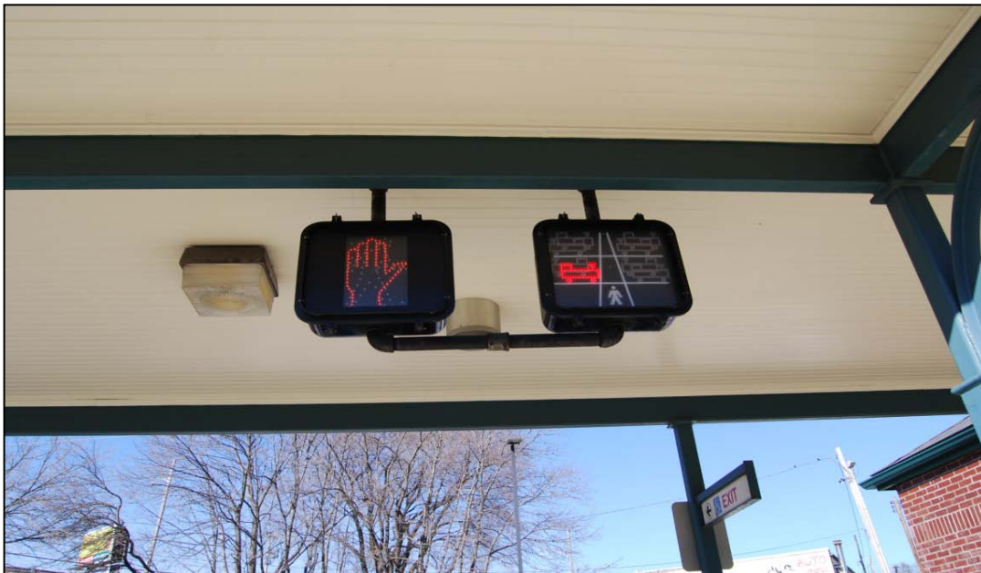
Figure 5: An example of a “Second train coming” display sign used on a passenger station platform.
